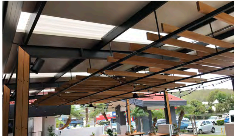
Coastal Blackbutt external ceiling screening. Coated Cutek Clear oil. Allows natural colour tones of the species to shine through.
